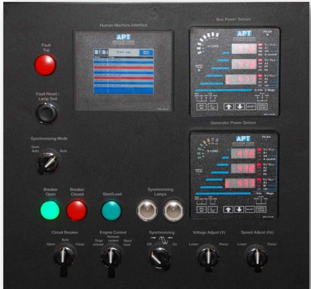
Figure 1: Automatic Paralleling Switchgear Control Panel Close-up
