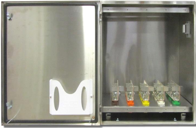
Figure 7: 800A Temporary Generator Quick Connection with Generator Signal Terminal Blocks for Customer Connections in Type 304 Stainless Steel Enclosure
