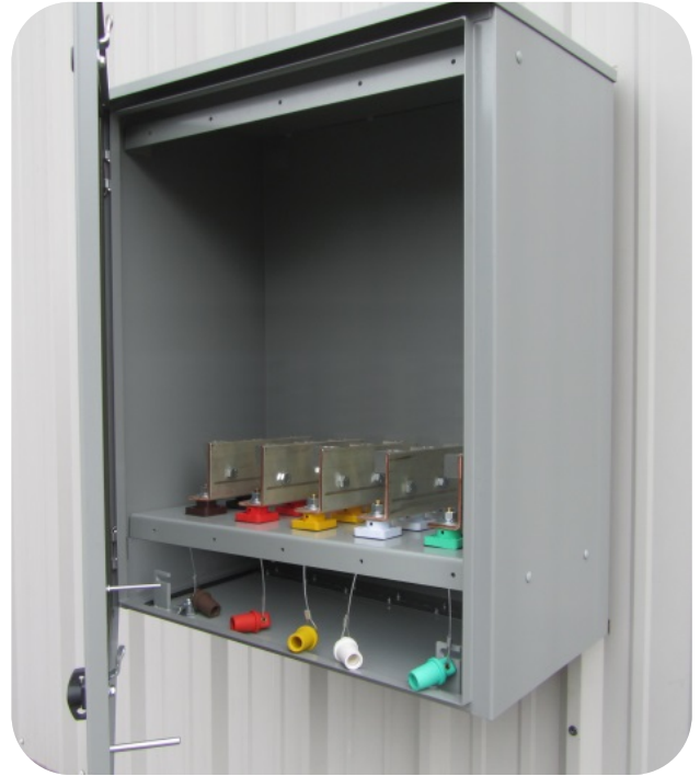
Figure 2: 1200A No Circuit Breaker (Inside Cover Removed)
