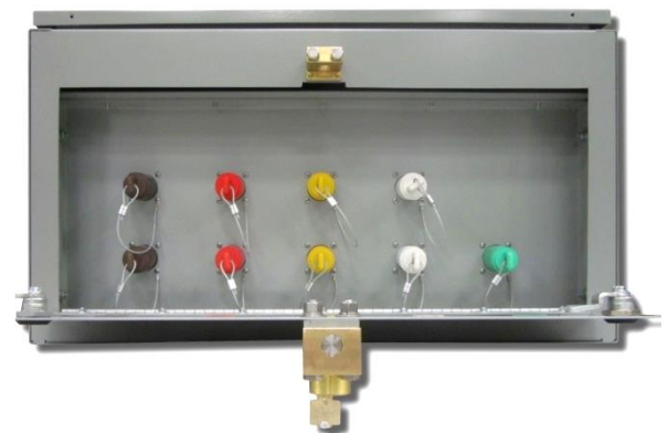
Figure 6: 800A Temporary Generator Connection Receptacles Accessed via Key Interlock with Utility Circuit Breaker
