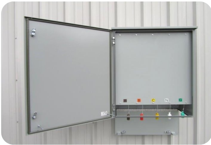
Figure 1: Carbon Steel NEMA 3R Enclosure Inside Access
