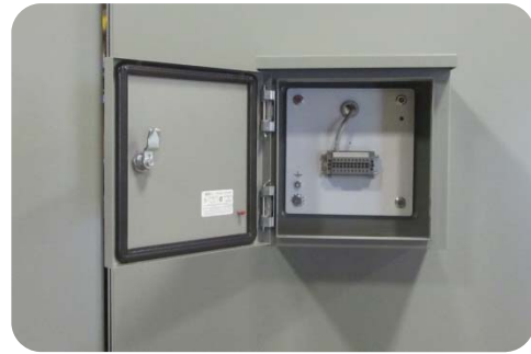
Figure 2: Isolated Customer Low Voltage Control Power Wiring Panel
