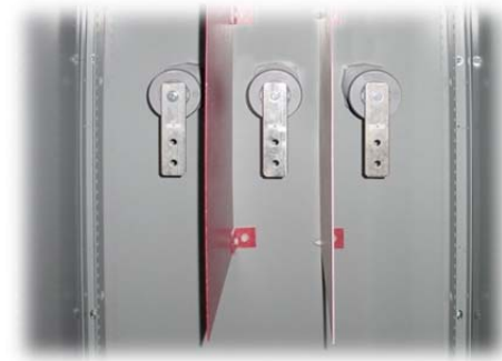
Figure 3: Rear view of 200A permanent connection with phase barriers
