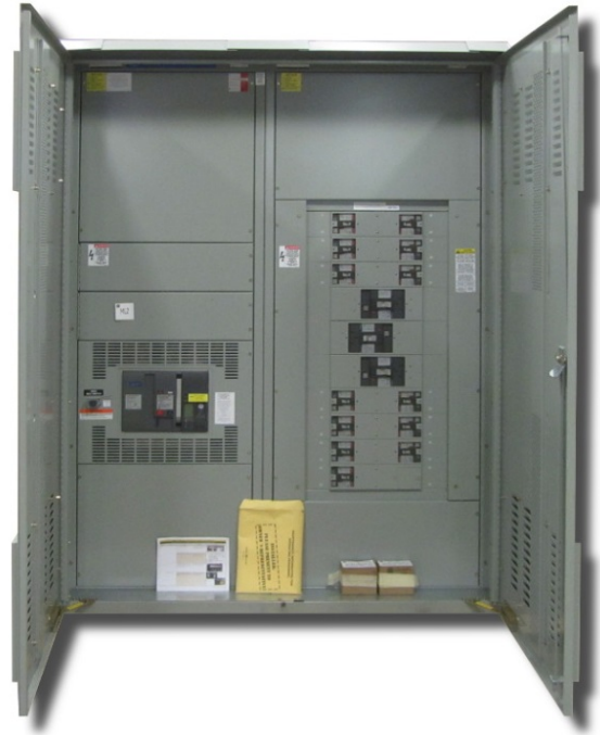
Figure 5: 2000A Solar Collector Switchboard
