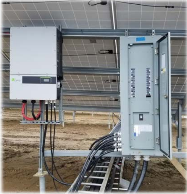
Figure 4: 600A Solar Combiner Panelboard
