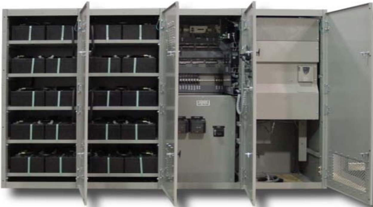
Figure 8: Solar Generated Power Battery Energy Storage System (BESS)
