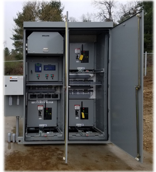
Figure 4: Inside Utility Intertie Protection & Generator Interrupter Switchgear
