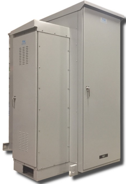
Figure 3: Utility Intertie Switchgear with Isolated Controls NEMA 3R
