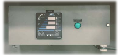
Figure 3: Power Quality Metering & Phase Rotation Indication
