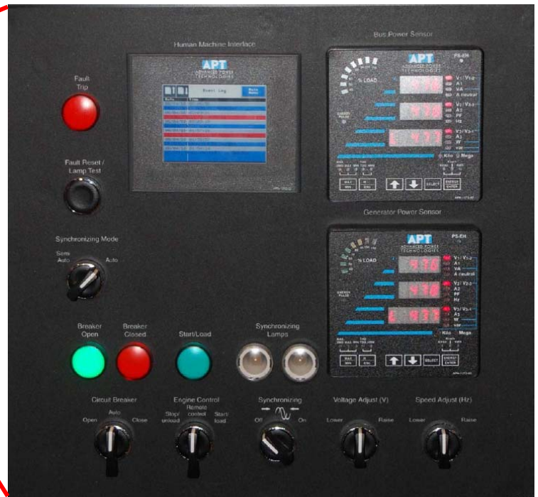
Figure 3: Close-Up Advanced Control Module for Generator Paralleling Control
