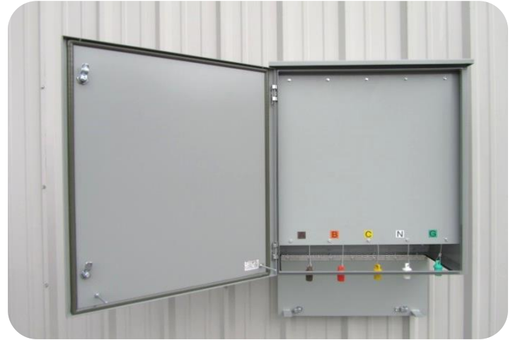
Figure 2: Loadbank Quick Connection Tap Box Inside Access Carbon Steel NEMA 3R
