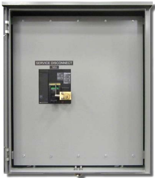
Figure 7: 800A Interlocked Utility Service Disconnect
