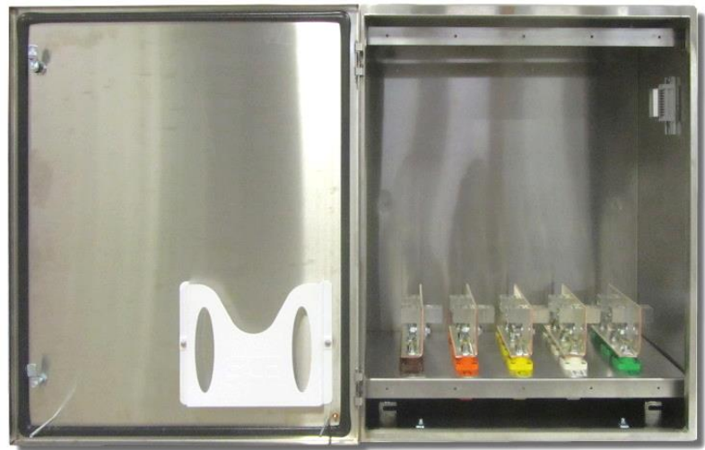
Figure 6: 800A Temporary Generator Quick Connection with Generator Signal Terminal Blocks for Customer Connections in Type 304 Stainless Steel Enclosure
