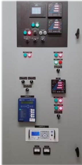
Figure 3: UP, PS, & ATC Control System Modules in Master Control Panel
