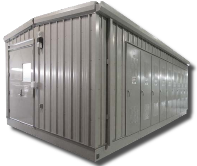
Figure 3: Outdoor Walk-In Medium Voltage Utility & Generator Paralleling Switchgear PwrHouse
