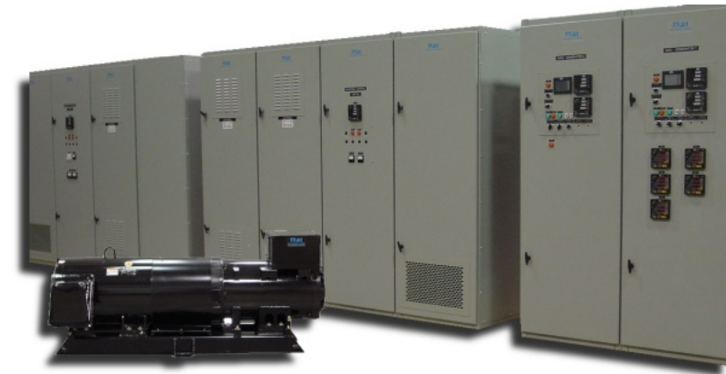
Figure 4: M-G Set, No Enclosure with switchgear control lineup
