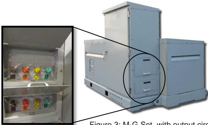
Figure 3: M-G Set, with output circuit breaker and quick connection receptacles in outdoor enclosure
