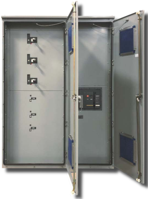
Figure 1: 2000A Microgrid DER Control Switchboard
