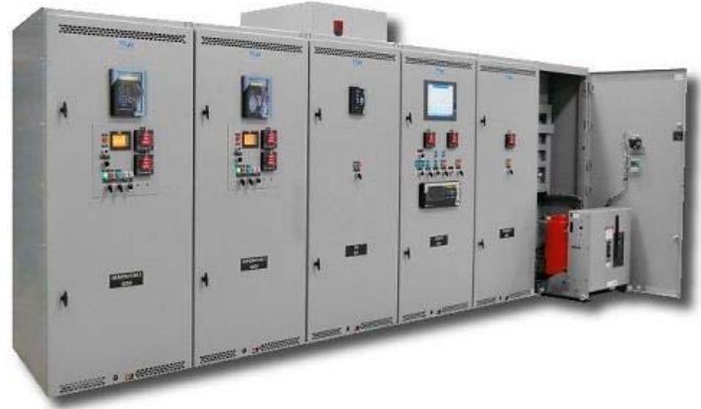
Figure 1: Medium Voltage Multiple Genset Utility Paralleling Lineup
