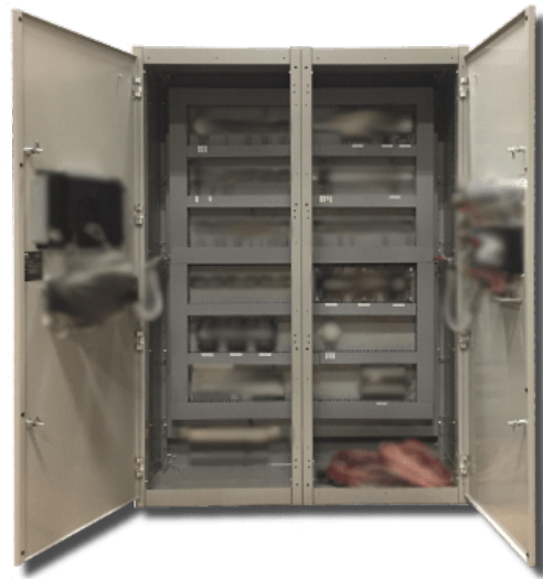
Figure 8: Generator Monitoring & Control Interior
