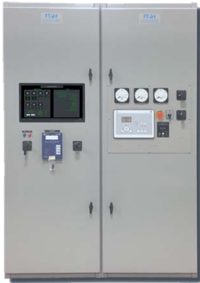
Figure 7: Generator Monitoring & Control Panel with Analog Metering, Protective Relays, & SCADA HMI
