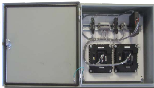
Figure 3: Two Generator Communication Conversion
