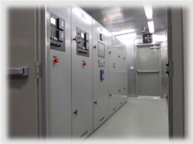
Figure 4: Inside Aisle of Low Voltage Utility & Generator Paralleling Switchgear PwrHouse
