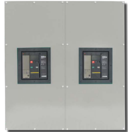
Figure 3: Partitioned with Two 1600A Insulated Case Circuit Breakers Panel
