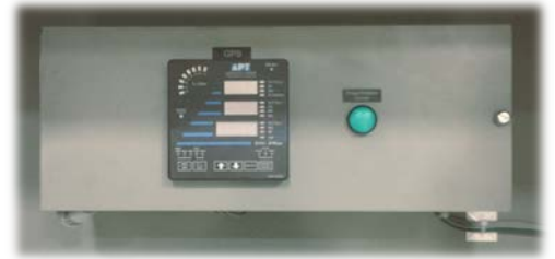
Figure 3: Power Quality Metering & Phase Rotation Indication
