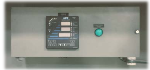
Figure 3: Power Quality Metering & Phase Rotation Indication
