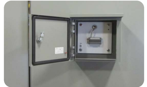
Figure 4: Isolated Customer Low Voltage Control Power Wiring Panel
