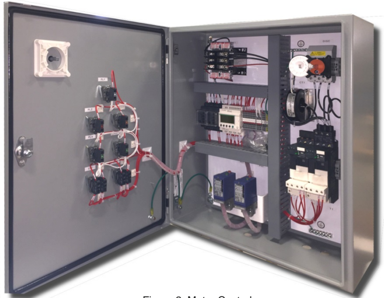
Figure 2: Motor Control & Annunciator Panel Interior NEMA 1
