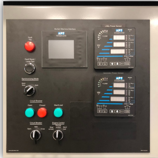
Figure 4: ATC - Automatic Closed Transition Transfer Control System Module with Operator Setpoints HMI & Source Power Meters
