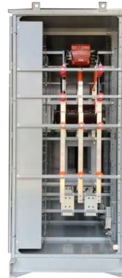
Figure 2: Automatic Transfer Switch Load Takeoff Section Access
