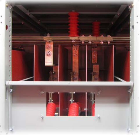
Figure 4: Main Bus with Visual Disconnect Window Removed
