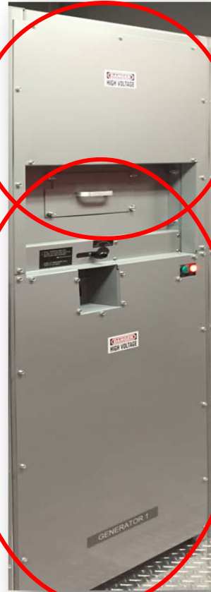
Figure 2: Single Front Access Section with Dead Fronts Attached
