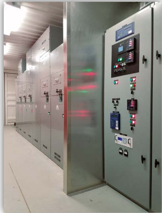
Figure 7: Front Access Switchgear, Isolated from Local and Remote Operator Control Stations
