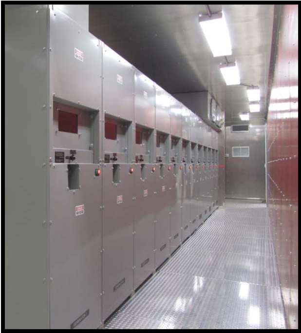
Figure 8: Inside of ISO Container based Switchgear Module with Ultra Compact Front Access (FA) Air Insulated Vacuum Circuit Breaker Switchgear
