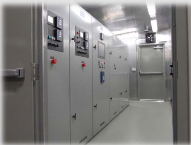
Figure 4: Inside Aisle of Low Voltage Utility & Generator Paralleling Switchgear PwrHouse
