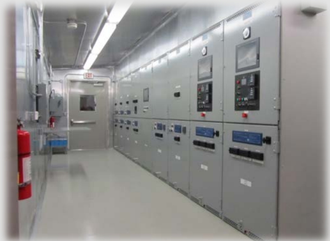
Figure 5: Inside Aisle of Medium Voltage Utility & Generator Paralleling Switchgear PwrHouse
