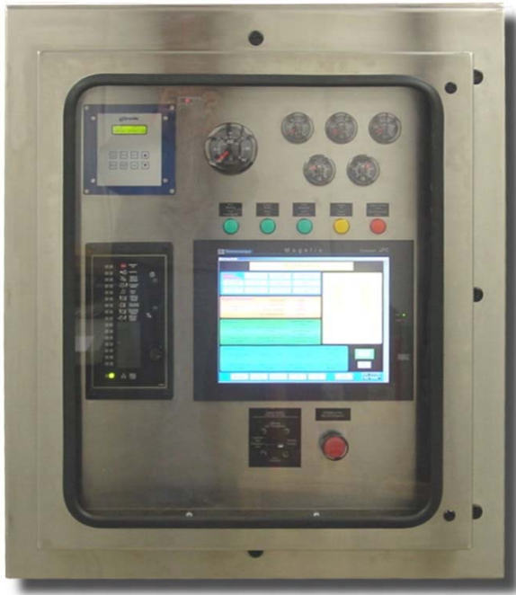
Figure 1: Digital Remote Annunciator & Control Panel 316 Stainless Steel NEMA 4X Enclosure
