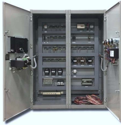
Figure 8: Generator Monitoring & Control Interior
