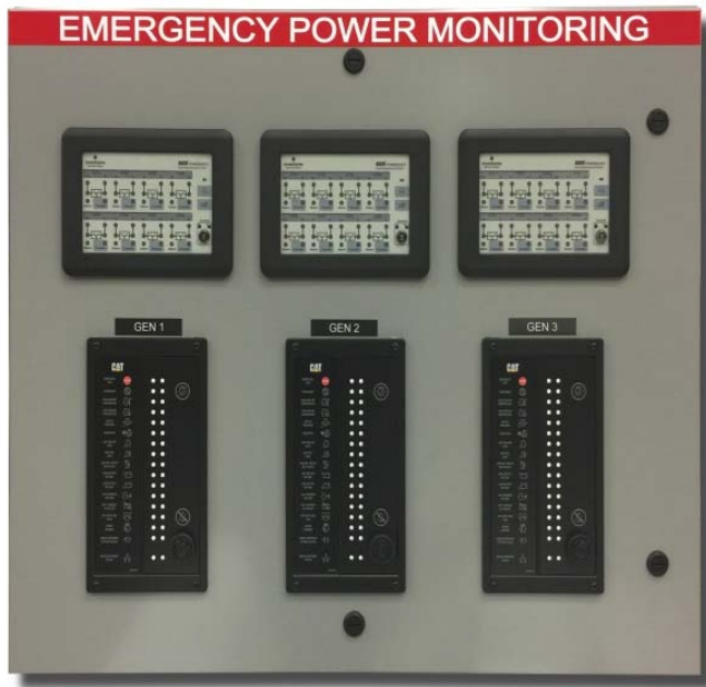
Figure 11: APT Emergency Power Monitoring Panel for Three Automatic Transfer Switches & CAT Generators
