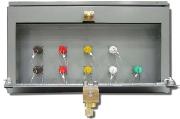
Figure 8: 800A Temporary Generator Connection Receptacles Accessed via Key Interlock with Utility Circuit Breaker
