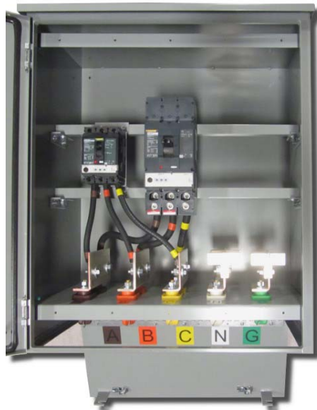
Figure 3: 600A Quick Connection with Auxiliary Circuit Breaker
