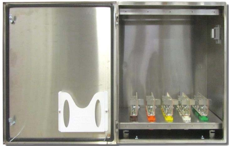
Figure 6: 800A Temporary Generator Quick Connection with Generator Signal Terminal Blocks for Customer Connections in Type 304 Stainless Steel Enclosure
