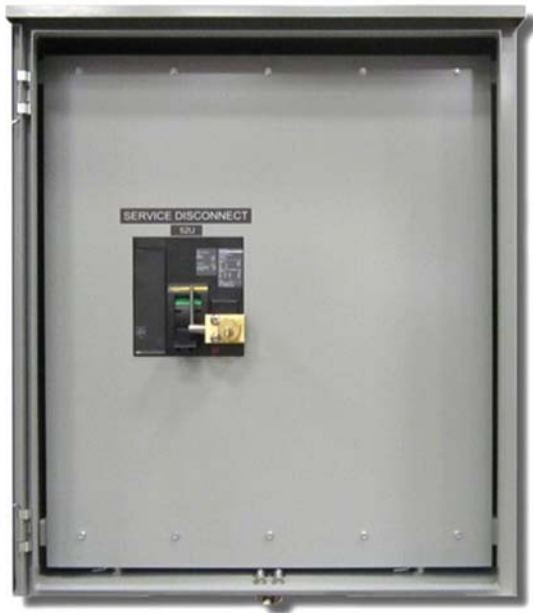
Figure 7: 800A Interlocked Utility Service Disconnect
